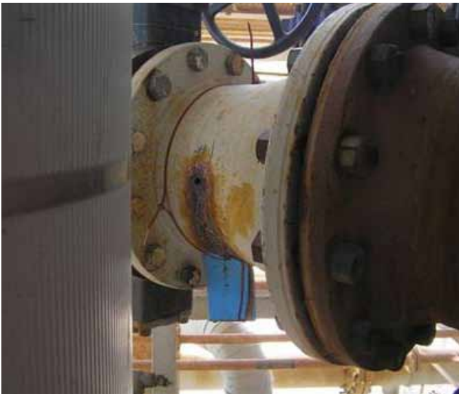
Appearance of a Leak
