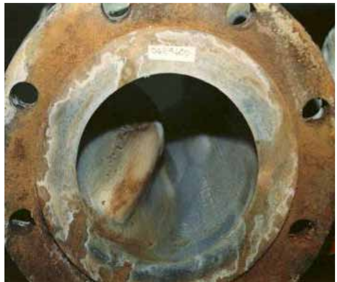
Single Lobe Liner Collapse
